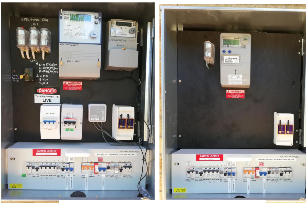
Spot the difference!! Our meter box with three-phase installed (on the left): single phase on the right
